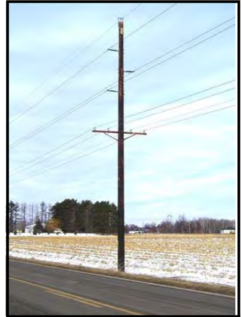
Typical 69 kV Transmission Line With Distribution Underbuild
