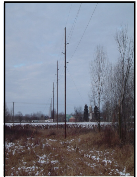
Typical 69 kV Transmission Line
