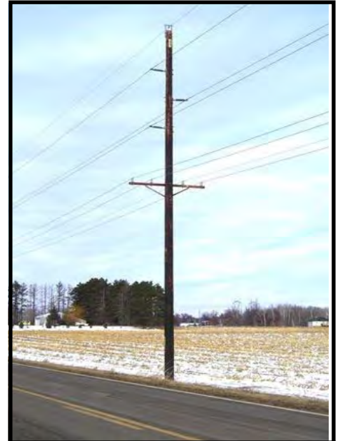
Typical 69 kV Transmission Line With Distribution Underbuild
