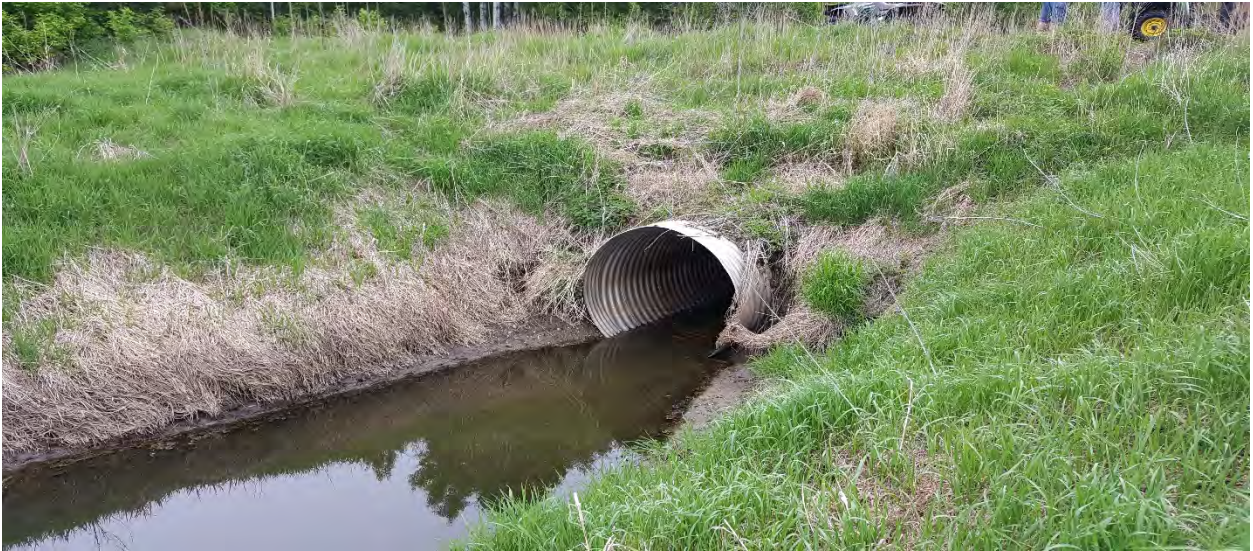
Inlet shot of railroad culvert. Outlet has almost no water coming out of it.
