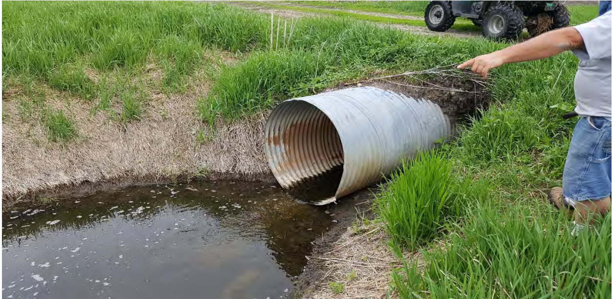
Culvert behind landowner's house. Eroding where the people are standing.
