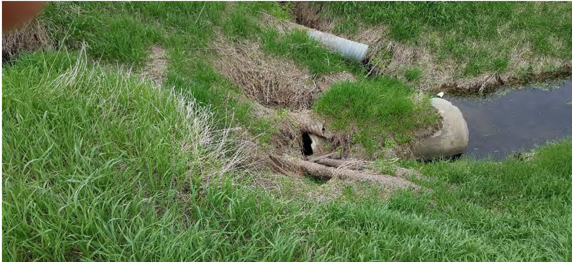
North side, cement culvert separating.
