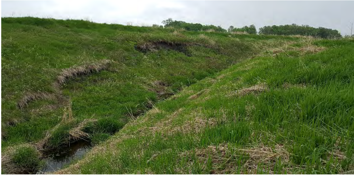
South Of 370 th St on Seneca land. Lots of sloughing.
