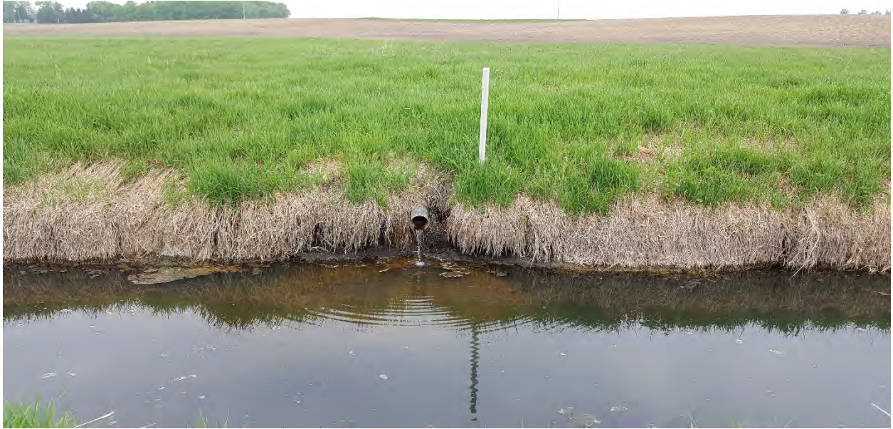
Another Tile from a basin project, (It is likely the historical water elevation of the ditch, prior to any excavating.
