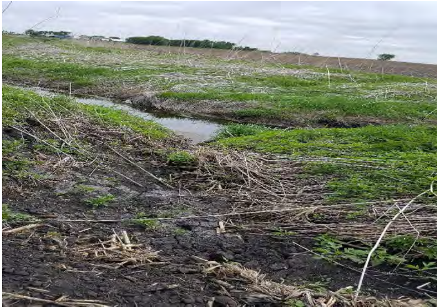
Sloughing which is causing a gully in the ditch bank.
