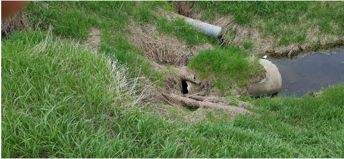
North side, cement culvert separating.
