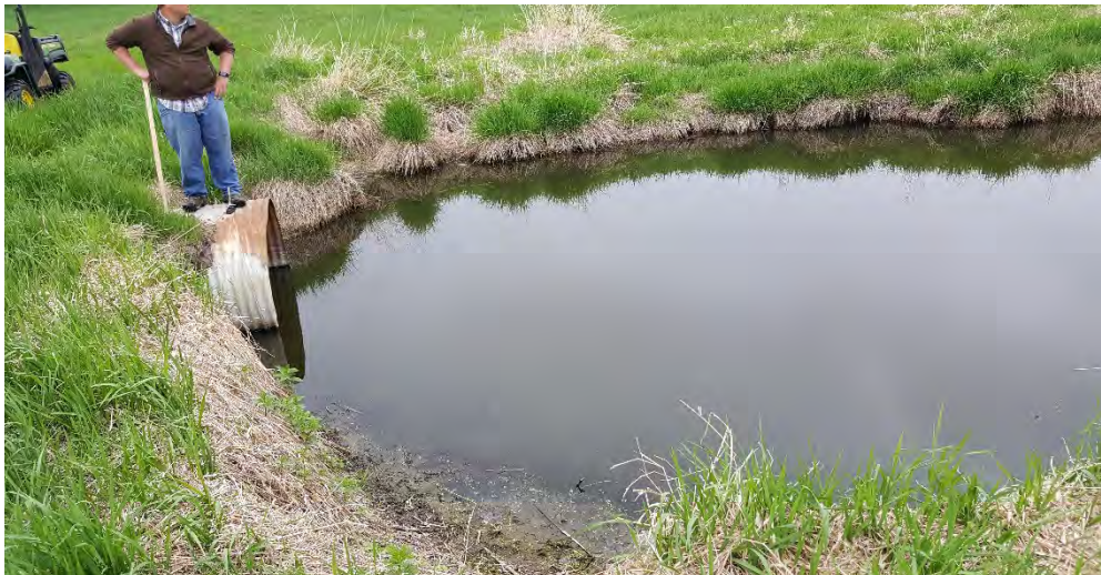
Ditch over excavated by culvert, Looks like pools on both sides.
