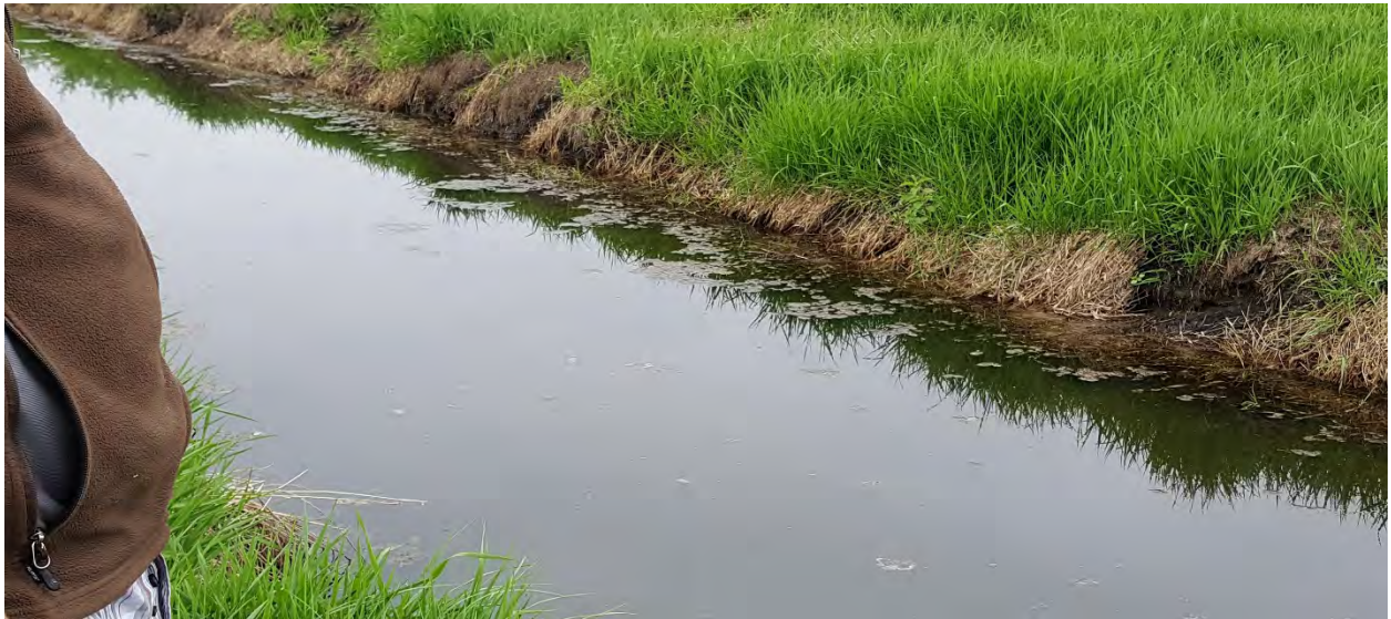
Sloughing from undercutting.
