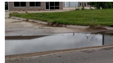
Standing water at property entrance along S. Webb Road
