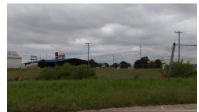
Damaged fence at stormwater catchment Source: Marvin Planning Consultants
