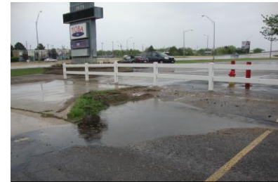
Standing water during a recent rain event
