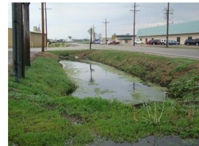
Standing water within one of the primary drainage routes
