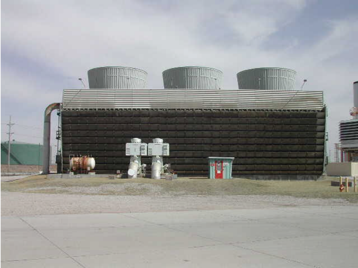
Figure 1: Existing Burdick Cooling Tower Built 1969
