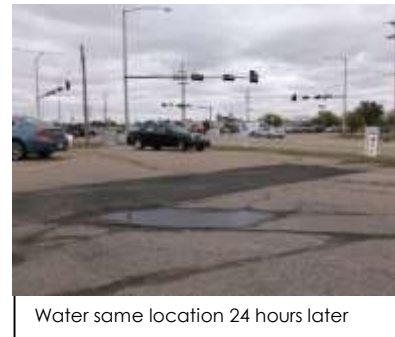
Standing water during a recent rain event
