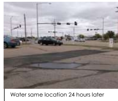
Standing water during a recent rain event
