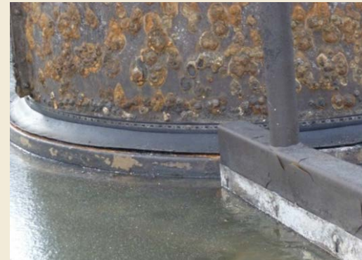
Corrosion in Clarifier
