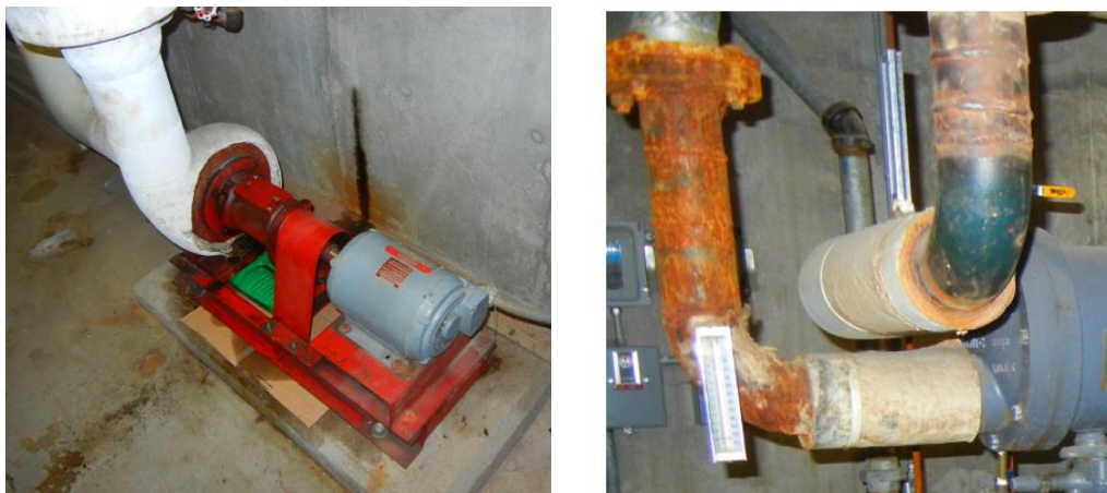
Hydronic Pump and Piping
