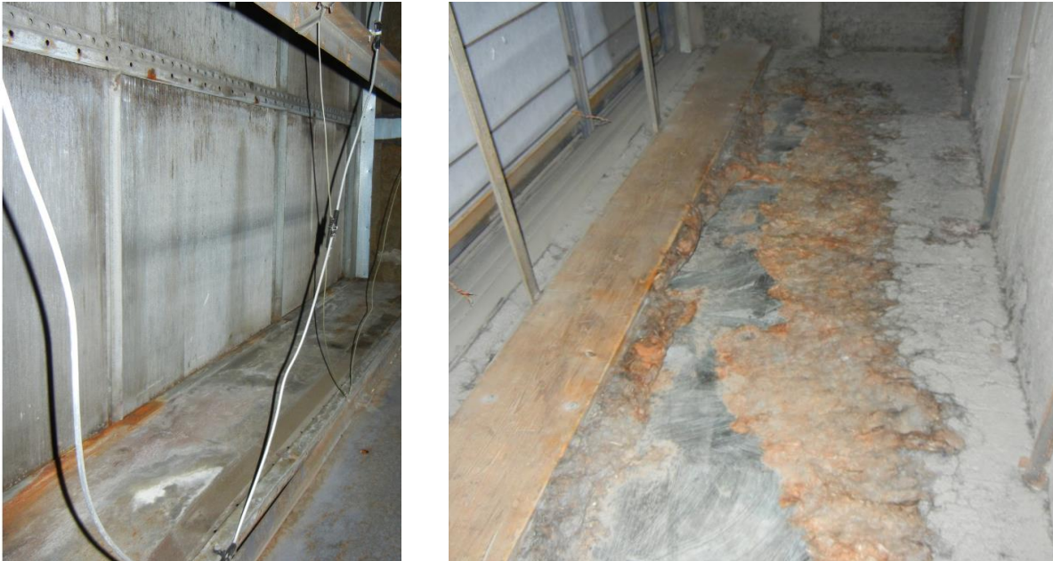
Multi-Zone AHU Interior Condition
