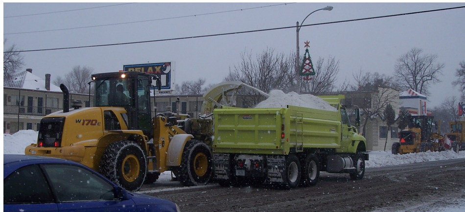
Snow Heaver driven by front of the loader blowing snow into the back of a dump truck.
