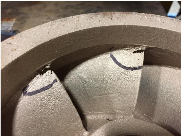
3. Heavy cavitation damage present on each of its vanes.
